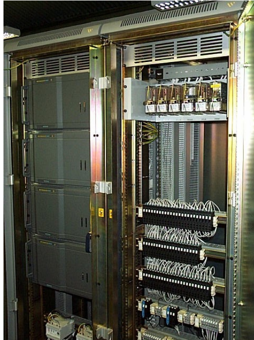
Figure 9.4: Westrace interlocking system. Photograph courtesy of Invensys Rail.
